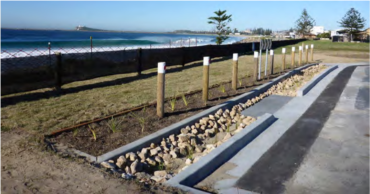
Figure 5-5 Installation of a constructed back-beach aquifer recharge trench at Stockton Beach, NSW (source: NSW State Government).
