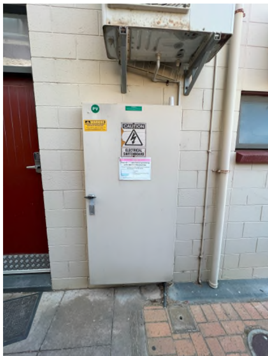
Figure 1 – Outside of Meter Box
